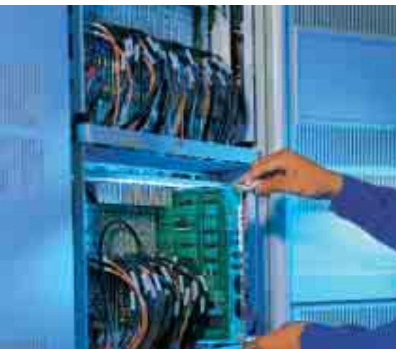
Hi-Tech Digital Network Infrastructure
