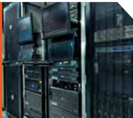
Data Centre and hosting services provided nationwide throughout Malaysia
